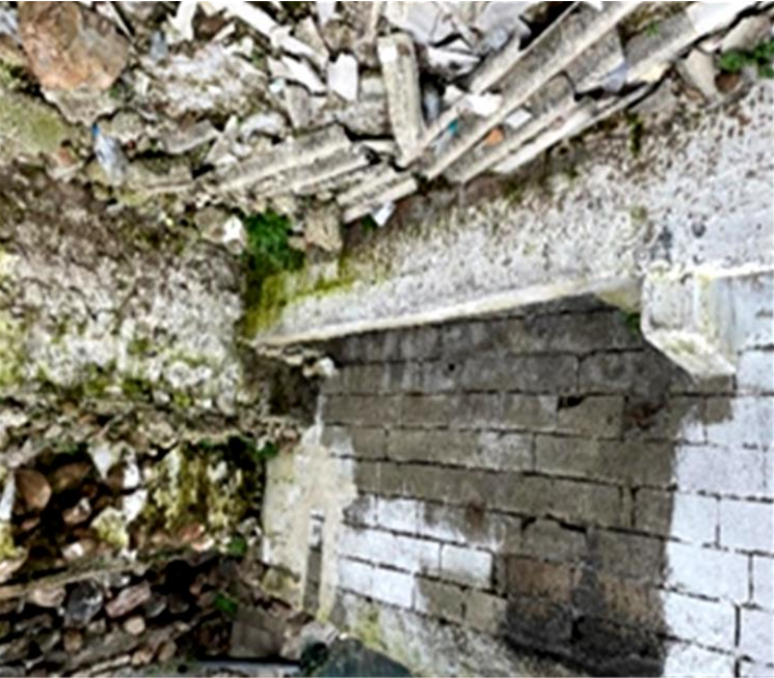
Image 5: Water Structure Turned into Ruins After the Earthquake
